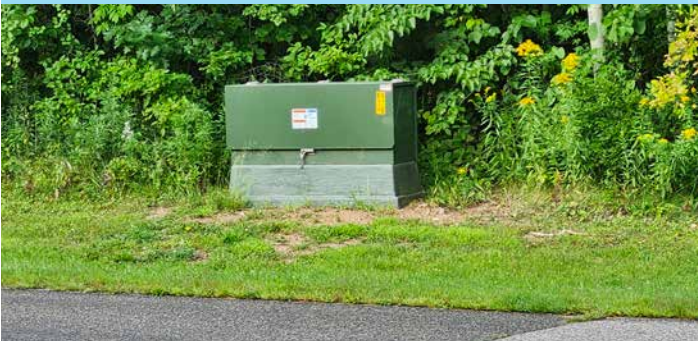
Figure 8. The power junction box brings three-phase power to the Mille Lacs Band of Ojibwe Department of Natural Resources campus, enabling EV charging infrastructure. Photo from Charlie Lippert, Mille Lacs Band of Ojibwe
